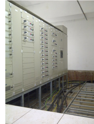
MCC Panels—New Plant
